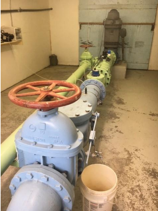
Figure 5: Typical drinking water treatment site for City of Yuma wells
